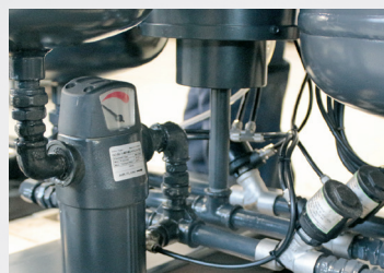
Air Filter - Pic. 5
